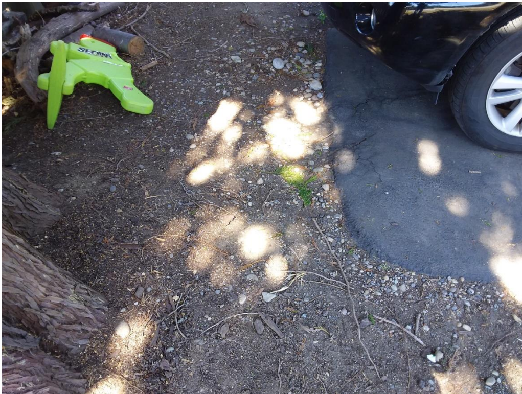
Figure 10. Photo of the base of the #1 tree showing the corner of the parking spot. Note the cracks indicative of root uplift.
